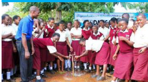
D&S engineer Samuel Kibet handing over a borehole installation at St. Marys's Kinyambu.
