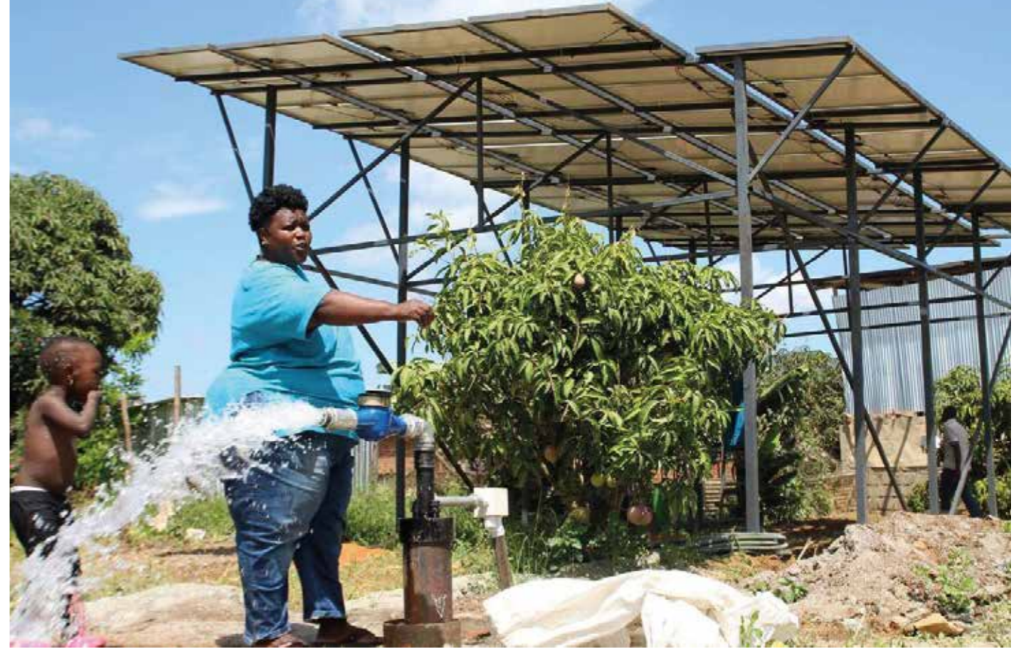
EMBU WATER PROJECT. SOLAR POWERED BOREHOLE PUMP INSTALLATION IN KANYIRIRI, EMBU. THE PUMP YIELDS OVER 70,000 LITRES OF WATER PER DAY FOR DOMESTIC AND FARMING USES (IRRIGATION AND LIVESTOCK).
